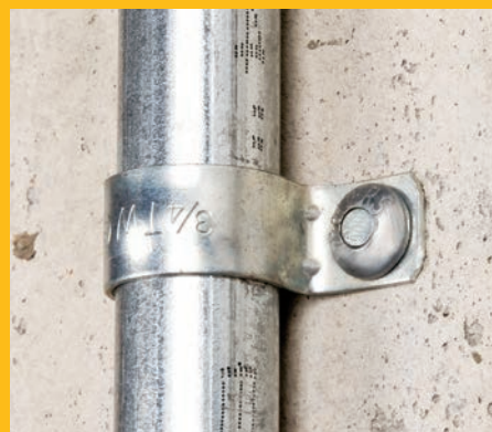
➤ Light duty electrical
